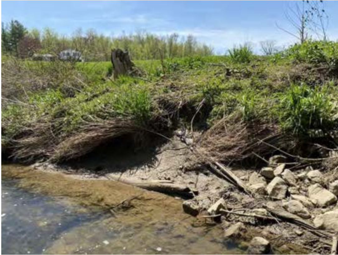
Photo 17 Looking at the right bank of watercourse and bank erosion
