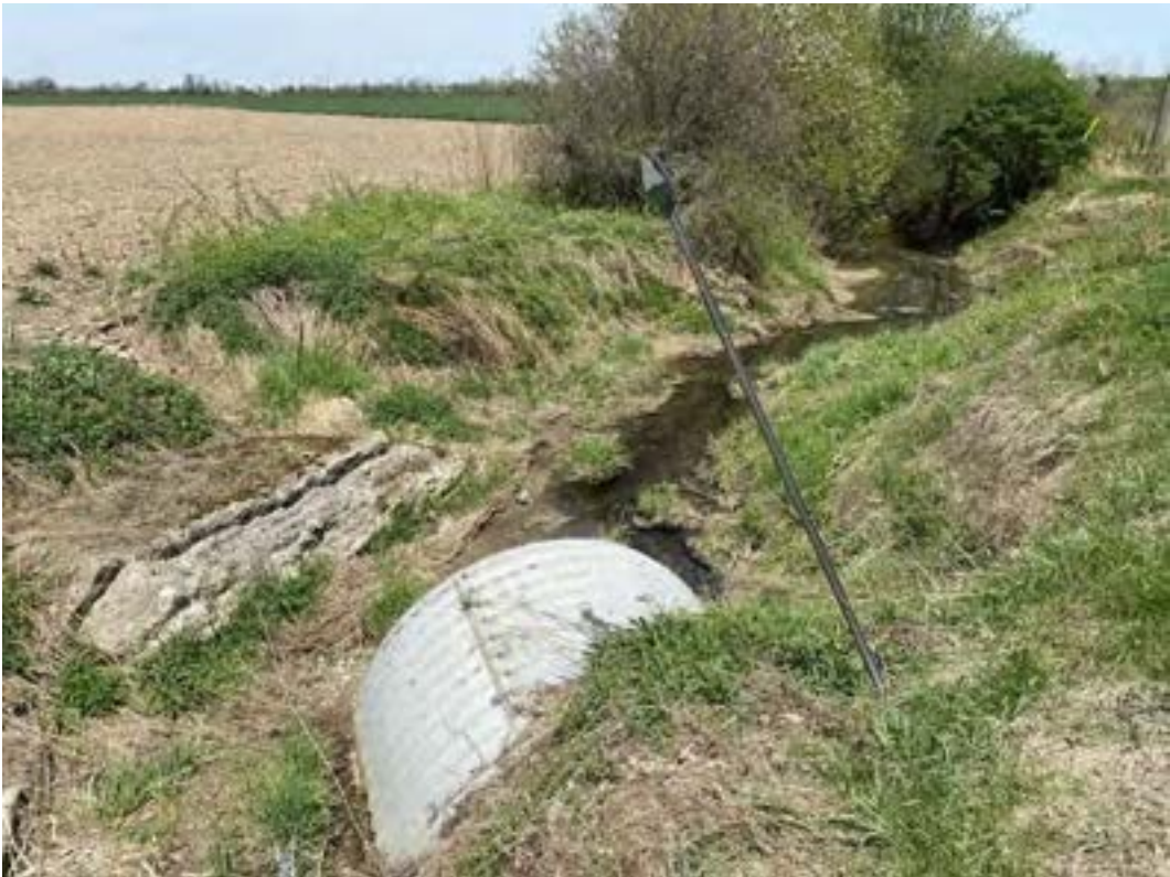
Photo 18 Looking northeast at the outlet of the culvert viewed from the ditch of the roadway
