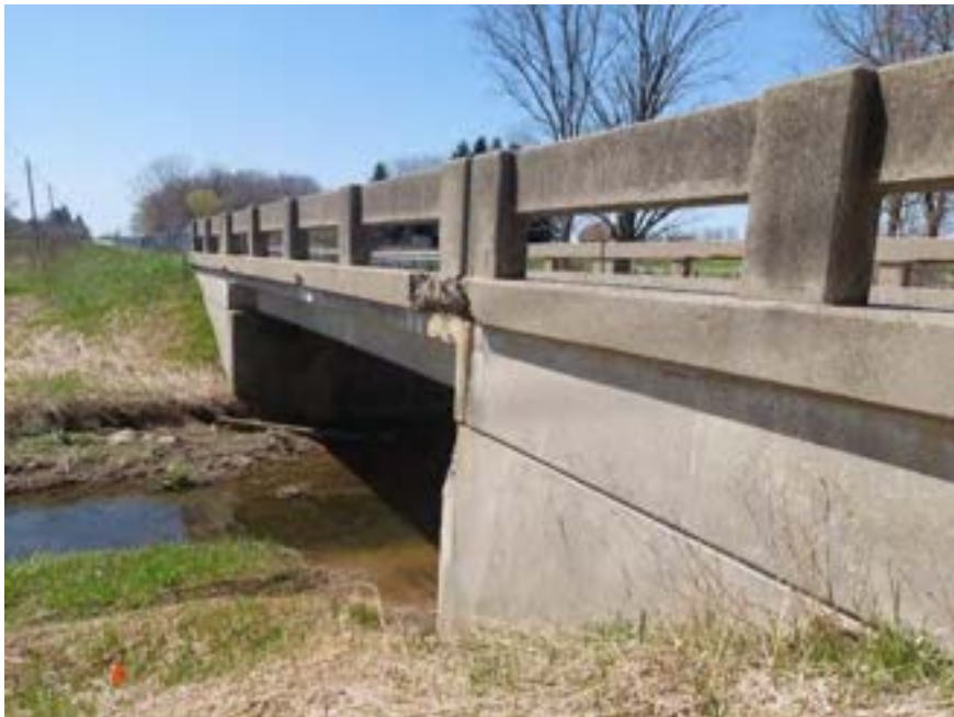
Plate 4: The concrete slab on precast T-beam bridge over Spittler Creek along Oxford Road 19, looking west.
