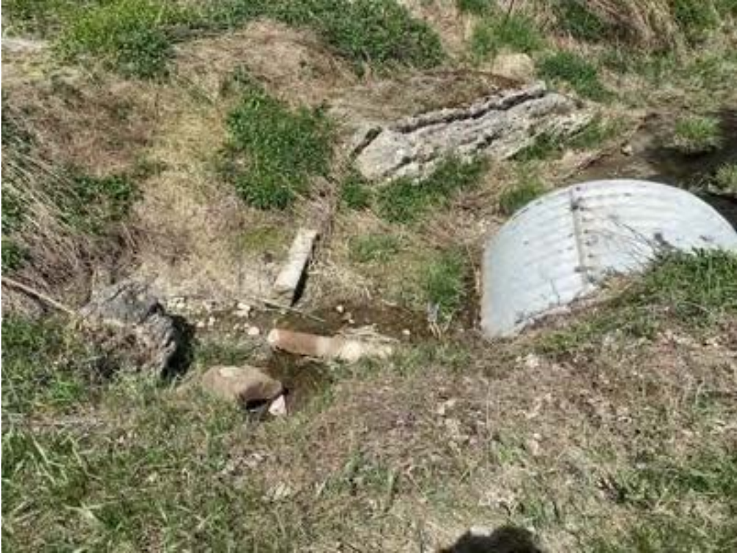
Photo 19 Looking down at concrete debris found in the ditch of the roadway
