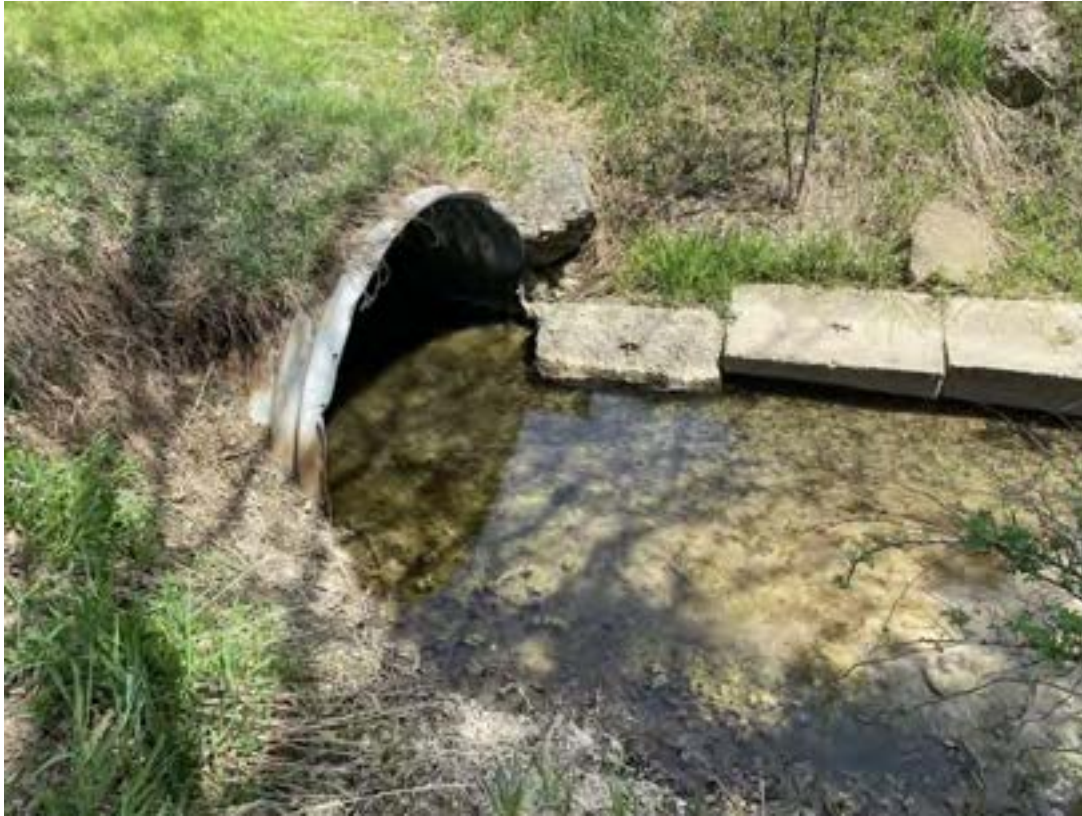
Photo 21 Looking down at the inlet of the culvert from the ditch of the roadway.
