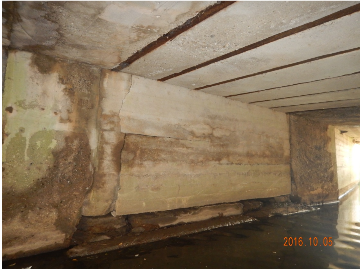
Image 4.0.4 Concrete Culvert with a BCI of 48.02 (Poor)
