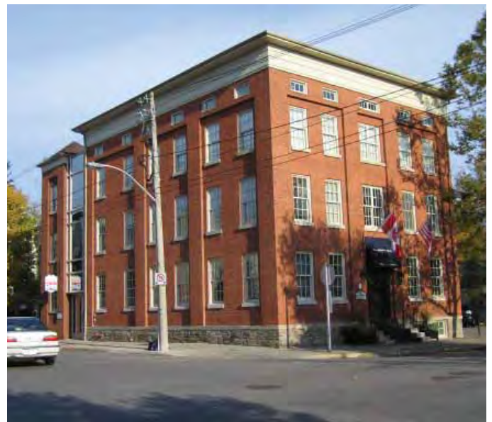
Cornices and parapets are often subjected to deterioration due to weather exposure.
