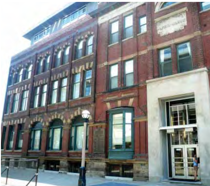
Where necessary, cornices and parapets should be repaired or replaced to their original configuration.
